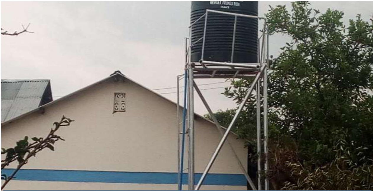
1000 LITRE TANK INSTALED WITH PROJECT FUNDS IN POSITION
